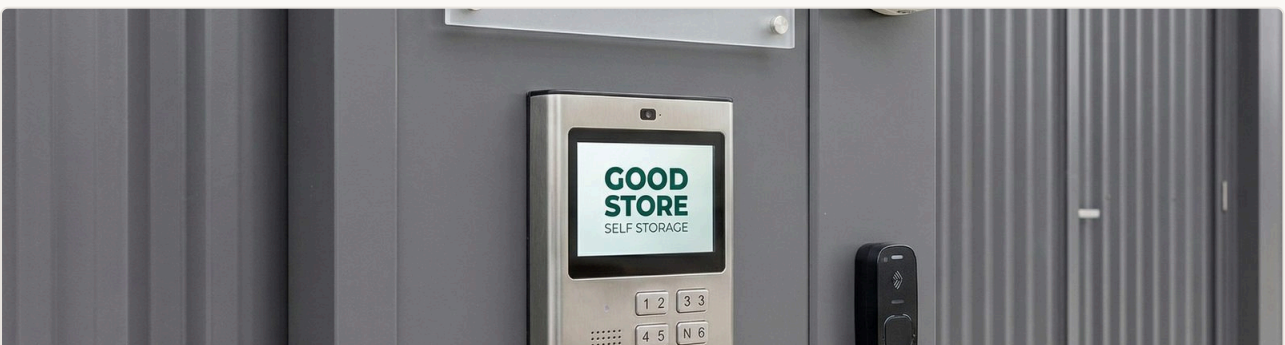
Secure 24/7 access with camera surveillance — standardised security infrastructure across modern facilities
